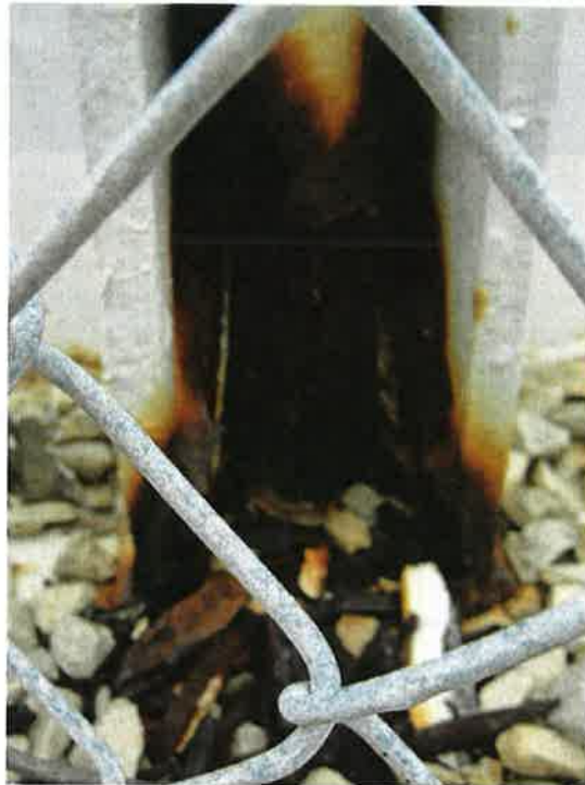
Anchor bolt in need of repair
