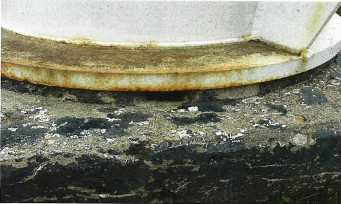
Foundation grout in need of repair
