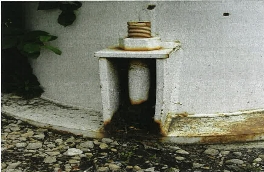
Anchor bolt in need of repair
