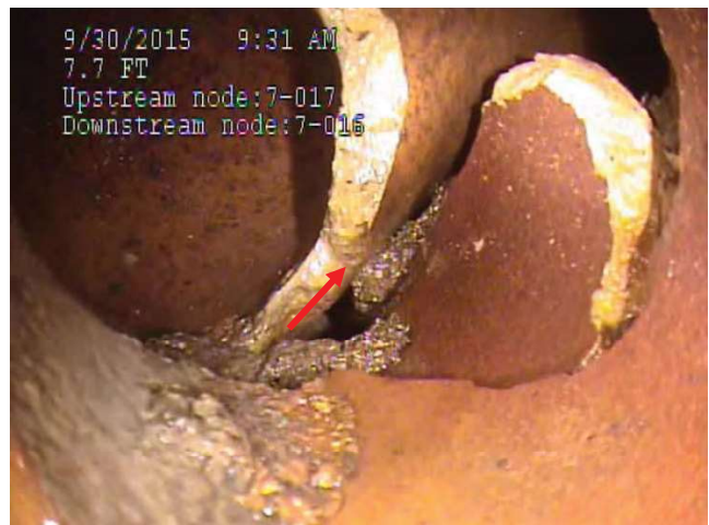
#5: Pipe Defect at 7.7 feet from MH 7-017 (collapsed existing lateral service)
