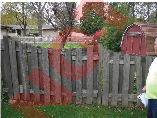
#5: Possible Access Route to PR from Frank St. looking North; Fences R&R-E of 931/935 Summit
