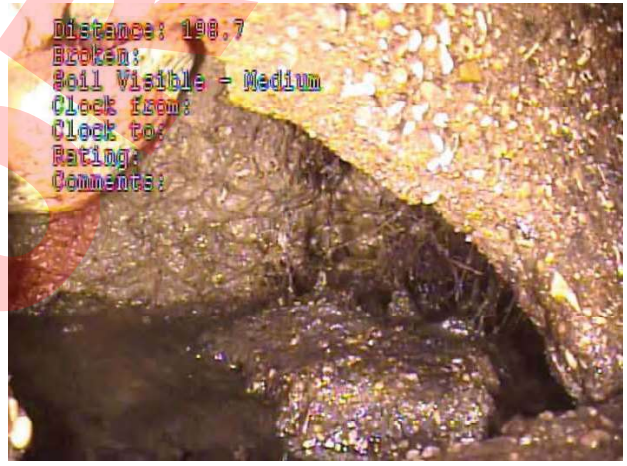
#4: Pipe Defect at 198.7 feet from MH 3-090 (Broken pipe, hole void visible)
