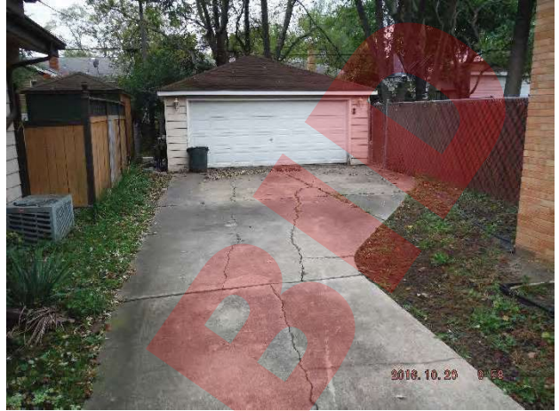
#2: End of Driveway (Possible Access Route) – Fence to be removed and re-erected (R&R-E)
