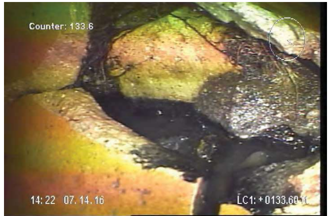
#6: Pipe Defect at 133.6 feet from MH 6-018 (tap break-in, hole void visible and fracture multiple)
