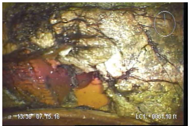
#6: Pipe Defect from 52.7 to 61.1 feet from MH 6-170 (Broken pipe)
