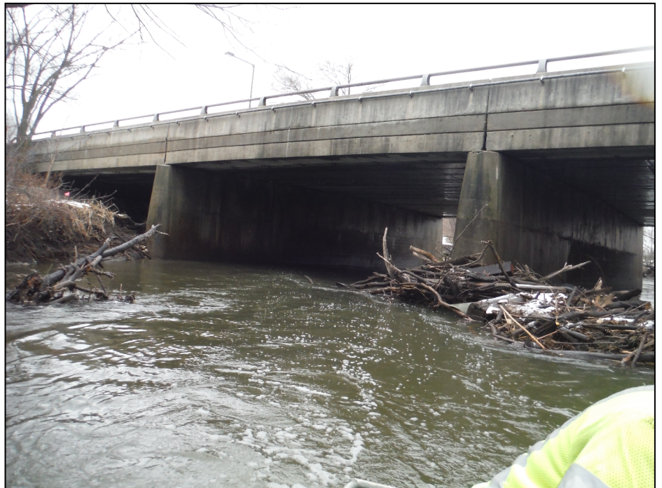
Photograph of upstream side of St. Charles Road Bridge, debris at west pier.
