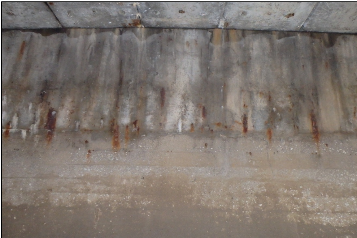
Photograph 14: View of Typical Concrete Condition of West Pier Extension on the West Face, Looking East.
